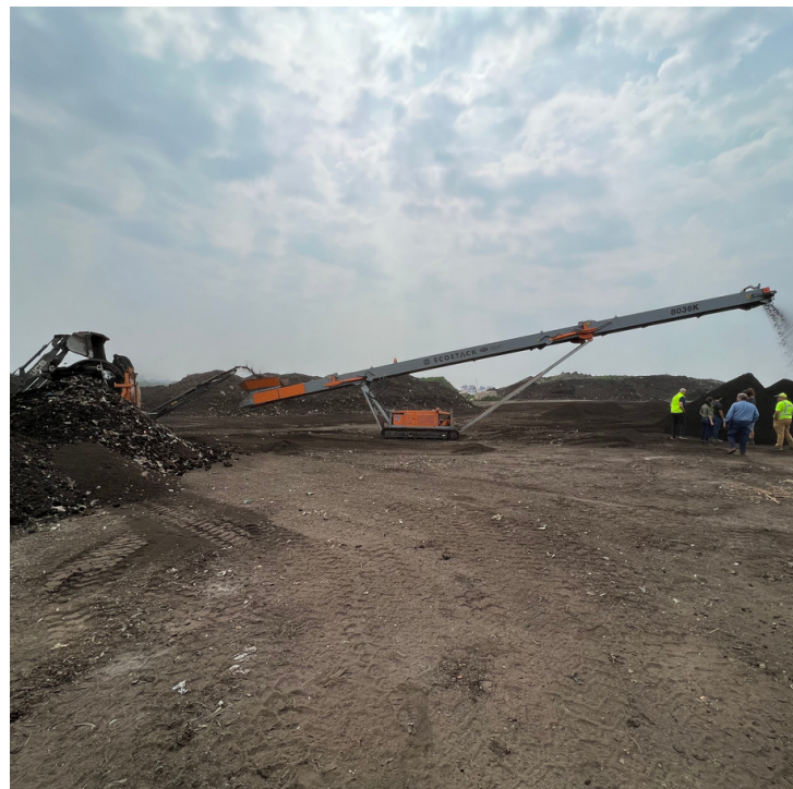
*Final processing stage of finished compost product at Whole Earth Compost Facility Photos courtesy of Andrew Meland
